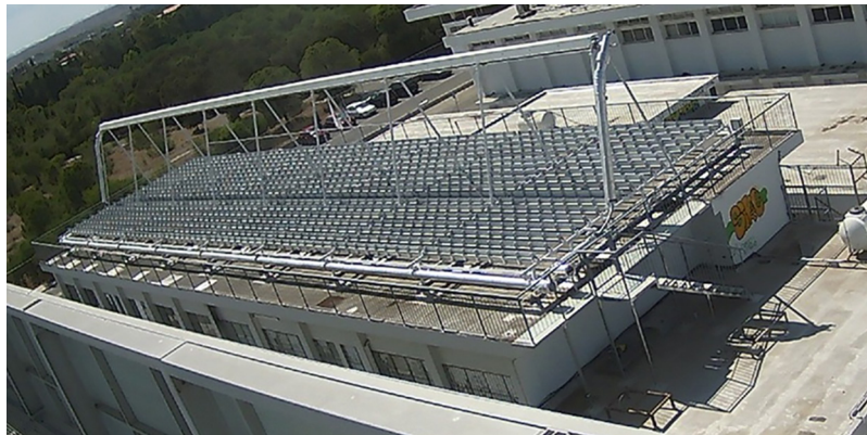
Fig. 10. Linear Fresnel Solar Collector.
