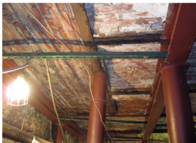
Figure 6: The general condition and configuration of the brick arches.
