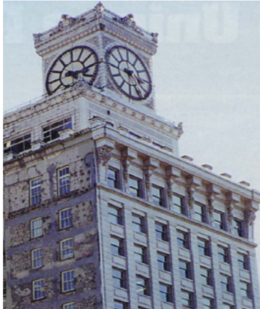
Figure 1: The north and west elevations of the Vancouver Block Building before the rehabilitation works.
