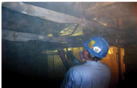
Figure 7: The application of shotcrete in an especially congested area of the basement behind the elevator shaft.
