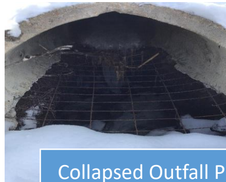
Separated Outfall Pipe
