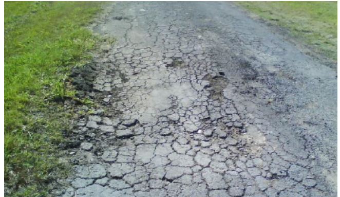
Deteriorated pavement with severe alligator cracking
