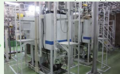
Floatation separation equipment
