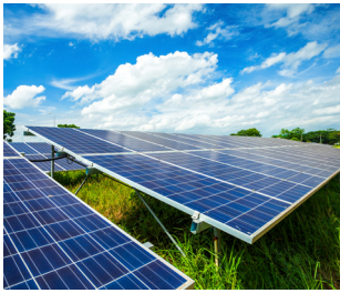
Solar and Battery
