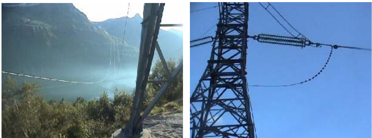
Figure 2. Left: Picture of the Glomfjord span. Right: Termination of fibre-optic cable with creepage extenders to ground potential.
