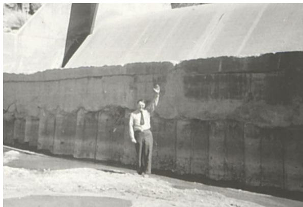
l. Channel degradation resulting from lack of upstream sediment source, downstream from Sumner Dam near Fort Sumner, NM.
