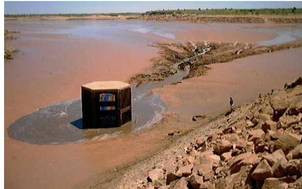
f. Reservoir sedimentation has buried the outlet at Summer Dam near Fort Sumner, NM.
