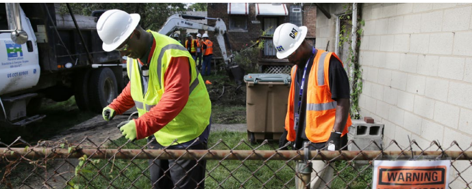
EPA contractors excavate contaminated soil in October 2016 at a home in the USS Lead Superfund site's zone 3 in East Chicago. Credit: Jonathan Miano — The Times of Northwest Indiana
