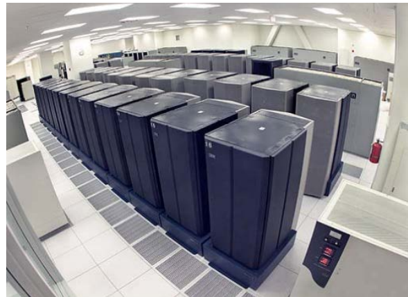
Figure 5-26. Typical Data Center
