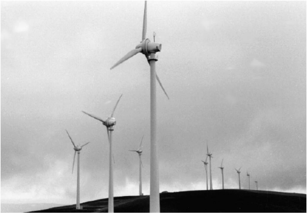
Figure 15.4 Edison Energie Speciali 10 MW windfarm at S. Giorgio la Molarra (20 wind turbines Enercon 500 kW)
