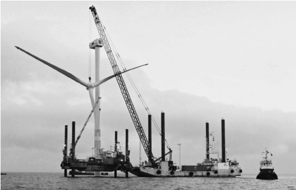
Figure 21.6 Utgrunden Offshore 10-MW wind farm
