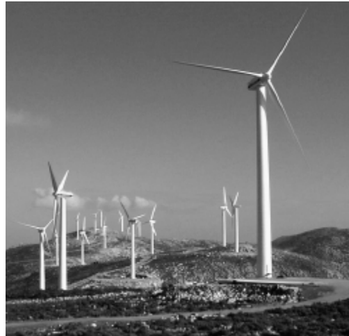
Figure 14.4 Windfarm with capacity of 11.2 MW on Evia Island, comprising 17 Vestas V42, 600-kW wind turbines (provided by G. Gilinou, CRES)
