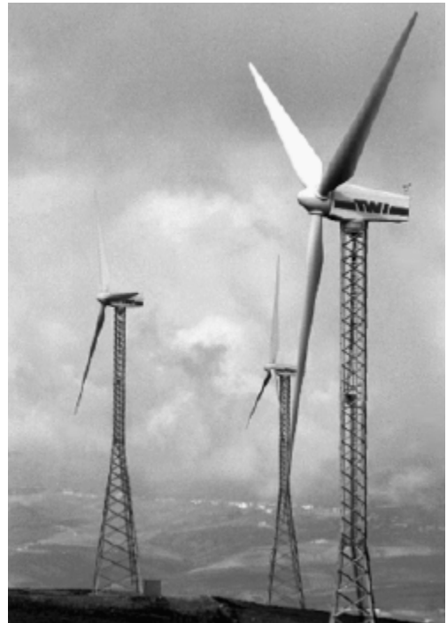
Figure 15.5 IVPC 4 27 MW windfarm at Bisaccia (12 wind turbines Vestas IWT 600 kW and 30 IWT 66 kW)
