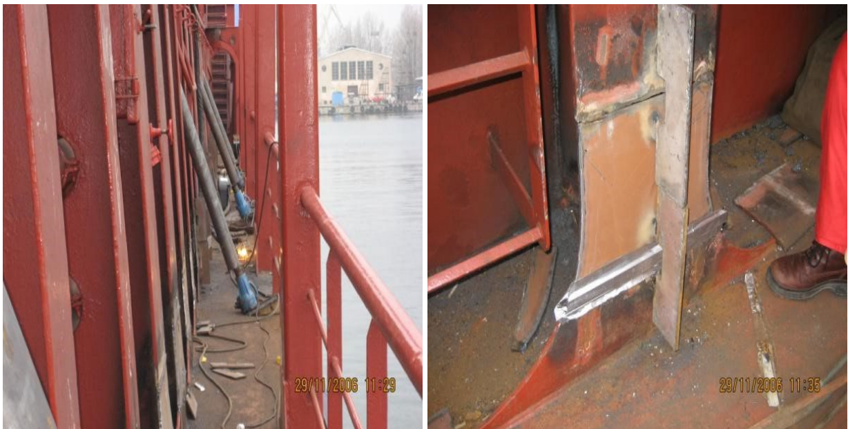
Figure 3 Return hatch coamings by the cut and welded additional part from coamings stool [5]
