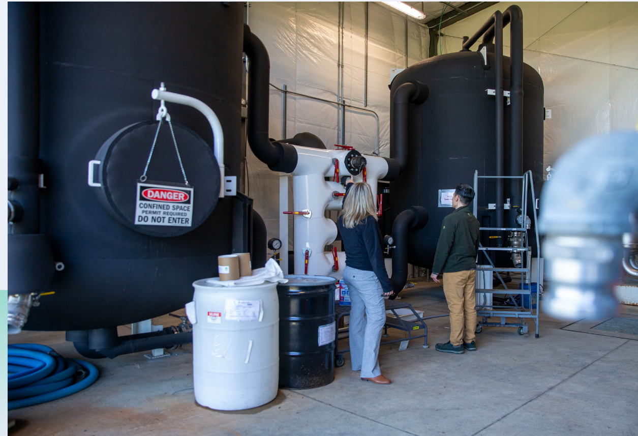
PFAS is removed from the Town's water supply wells by a treatment system constructed and operated by NASA.
