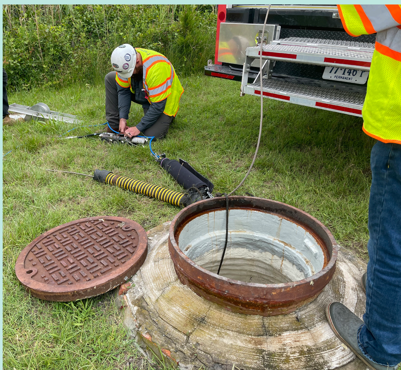
Workers repair the Island manhole and pipe that reduced PFAS concentrations entering the Wallops wastewater treatment plant by 80%.
