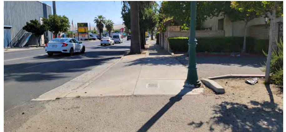
Sidewalk maintenance needed in various sections
