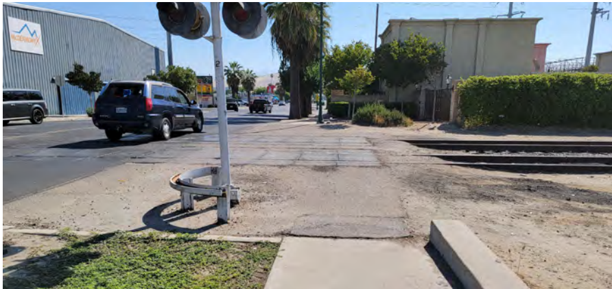
Sidewalk maintenance needed over at-grade railroad crossing
