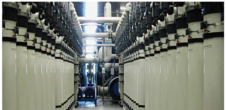
Figure 2. Photograph of two UF skids. Courtesy of VWS Deutschland GmbH – BERKEFELD
