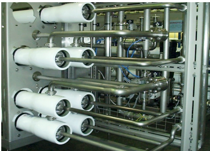
Figure 4. Photograph of an RO rack. Courtesy of WWS Deutschland GmbH – BERKEFELD
