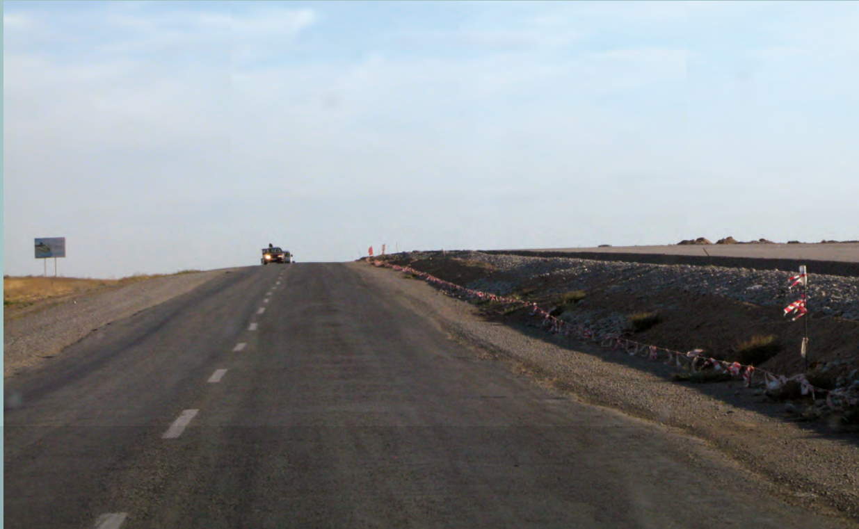
Kazakhstan: South-West Roads: Western Europe—Western China International Transit Corridor— section of the road being widened
