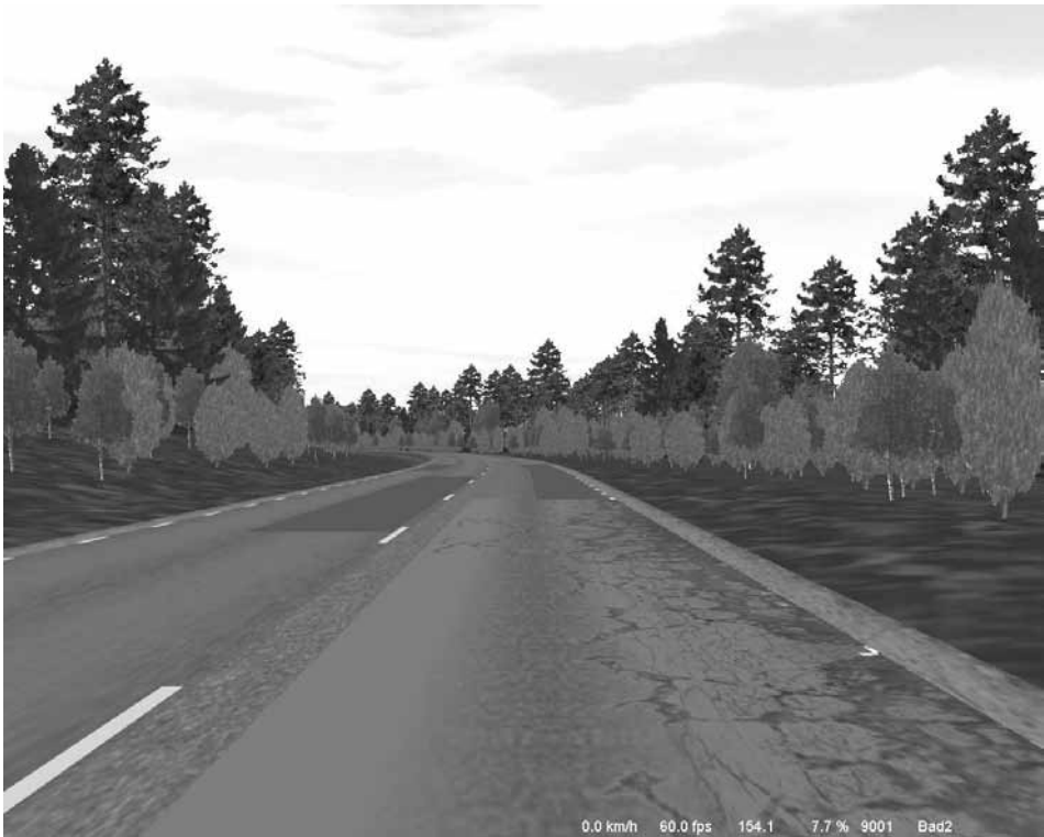
Figure 5. Example of a road with cracks and patches
