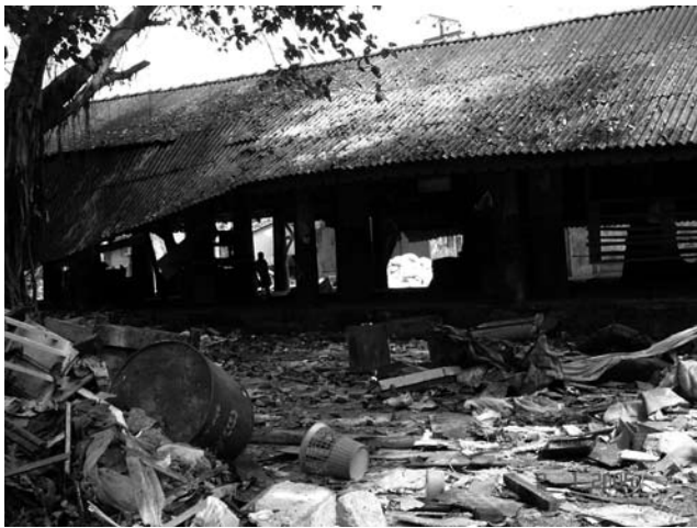
Fig. 1 The roof of the 18th c. market in the Old City of Galle caved in during the tsunami on 26 December 2004
