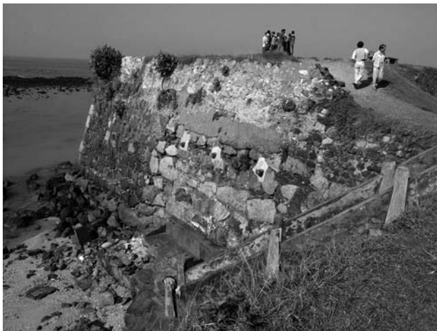
Fig. 5 Damage to rampart wall near Akersloot Bastion in Galle Fort
