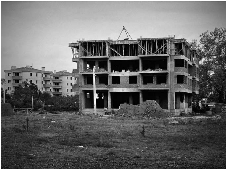
Fig. 11 Typical Turkish reinforced concrete building under construction showing installation of the hollow block infill (photograph © Randolph Langenbach)
