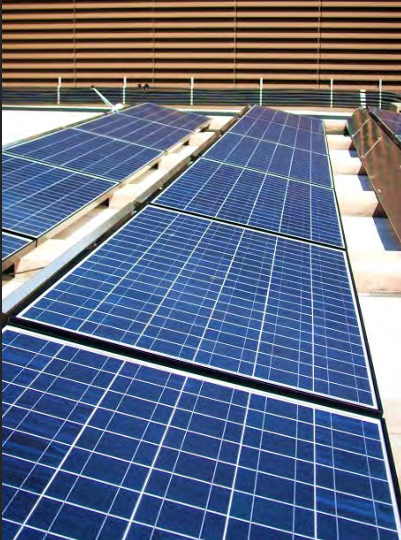
Figure 13: Thomas P. O'Neill, Jr. Federal Building Solar Boston, MA
