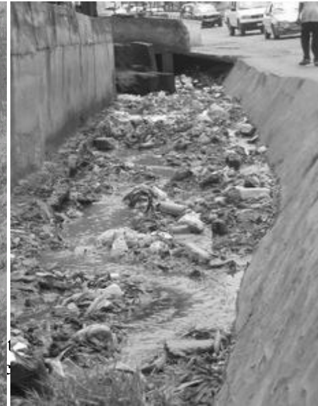
Figure 14: Clogged gutter in Accra
