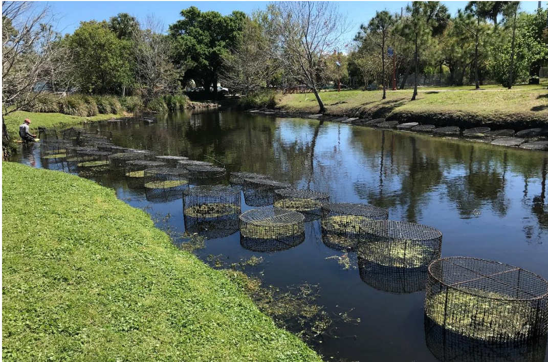
Figure 4. Final installation of enclosures along Moore's Creek, on both sides of the creek. Combined with past plantings, this area should grow and expand quickly.
