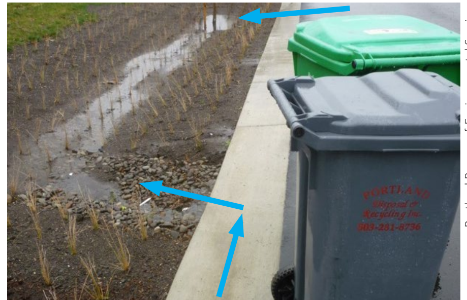
A valley gutter concentrates sheet flow from upstream and can cause localized deposition of debris as it flows into a bioswale in Portland, OR.
