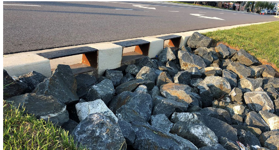
Wheel guards are installed over inlets that are parallel to traffic, such as on this median bioswale in Prince George's County, MD.
