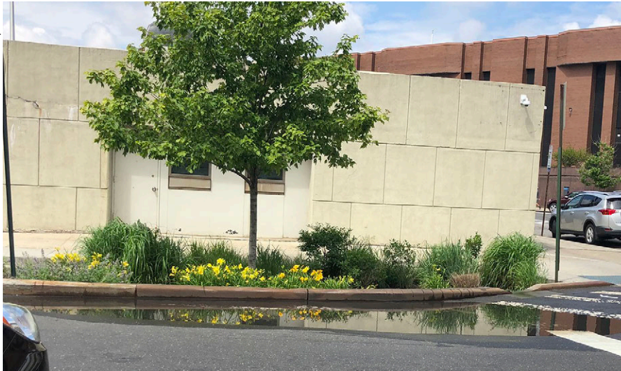
Poor grading allows water to build up on the road adjacent to a bioretention practice.
