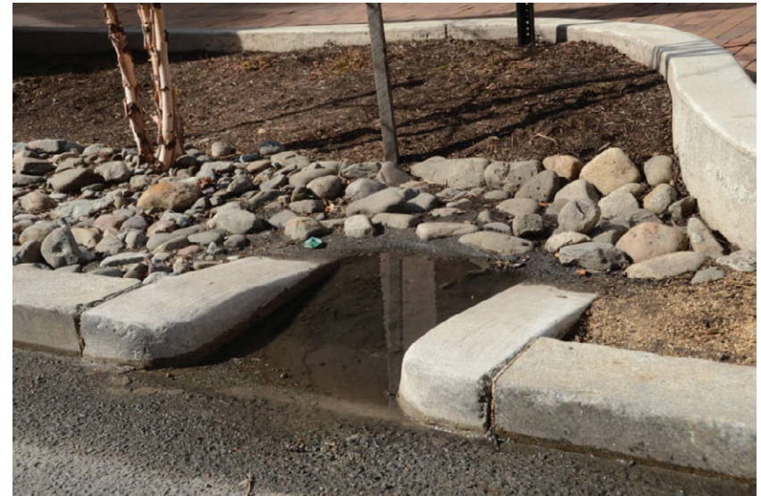
Incorrectly installed inlet.
