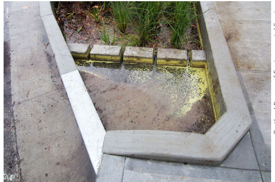
A concrete pad in a stormwater curb extension system in Portland, OR.
