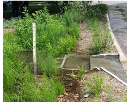
Utility Box Forebay (City of Omaha)
