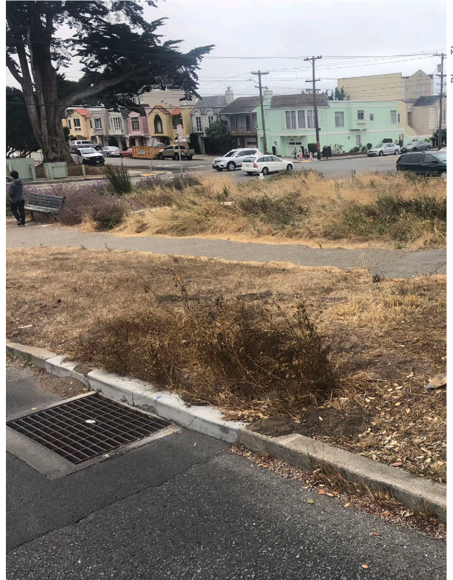
A pipe conveys runoff from a depressed drain to a bioretention facility in San Francisco, CA.
