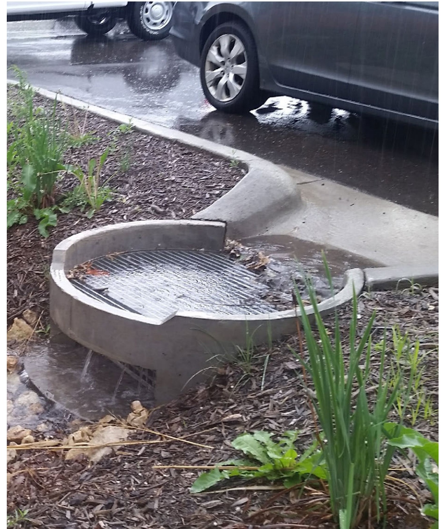
Proprietary inlet sump in Minneapolis, MN.
