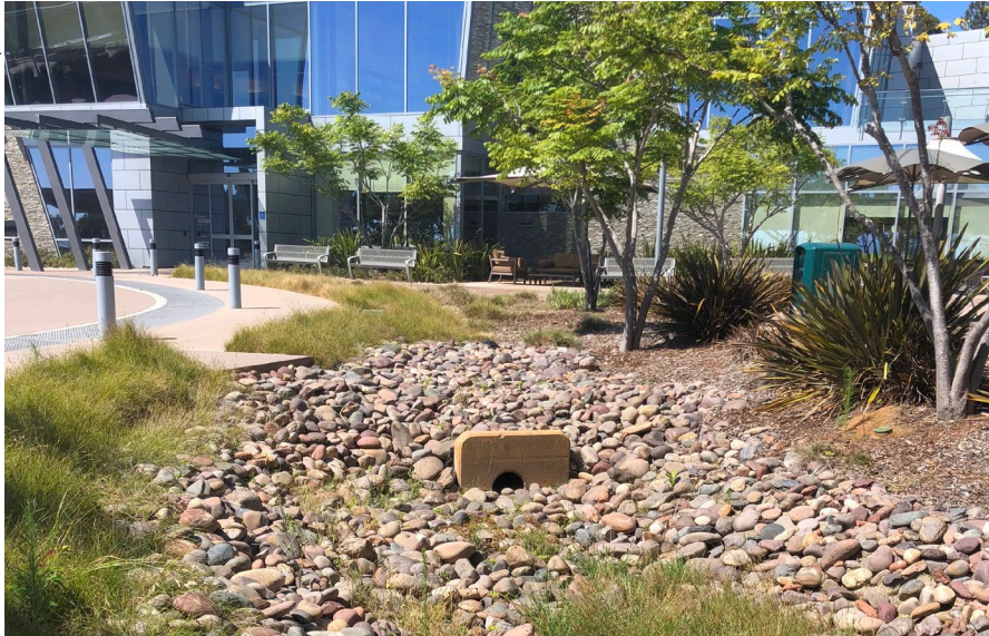
A pipe conveys and discharges roof runoff in San Diego, CA.
