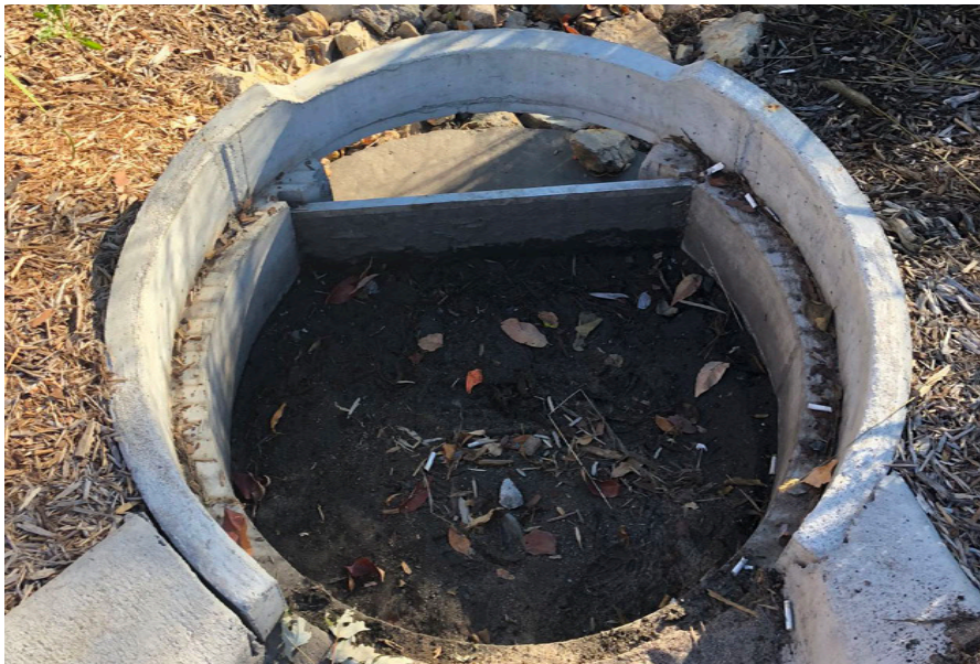
Pretreatment maintenance often requires removing the grate and scooping out sediment and debris for disposal off-site.
