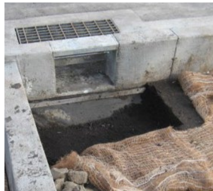
Depressed Drain (Portland Bureau of Environmental Services)
