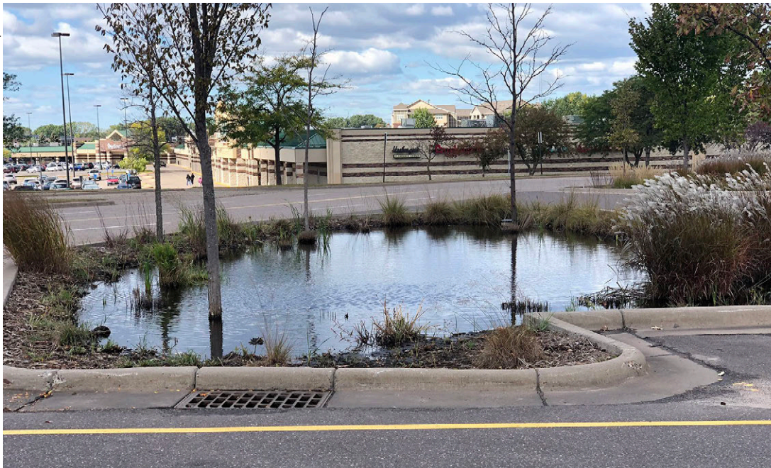
Ponded water remained for days after a storm, indicating poor drainage due to soils or outflow design.
