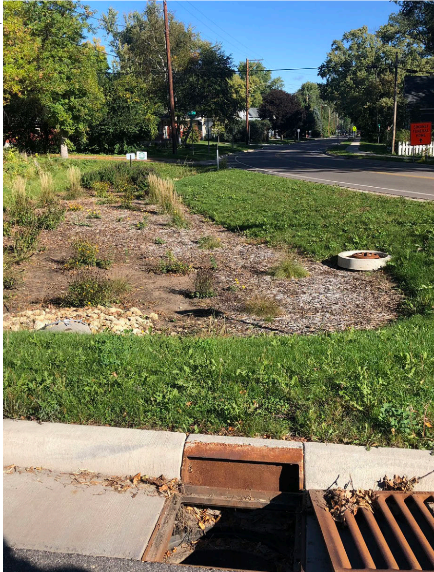
Water flows into a depressed drain and through a pipe to a bioretention facility in Minneapolis, MN.
