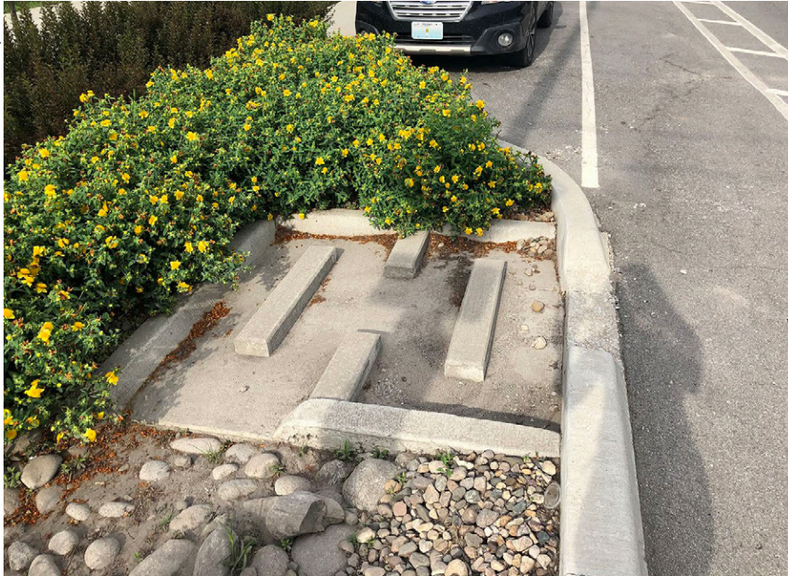
A concrete splash pad is paired with a stone forebay in Kansas City, MO.
