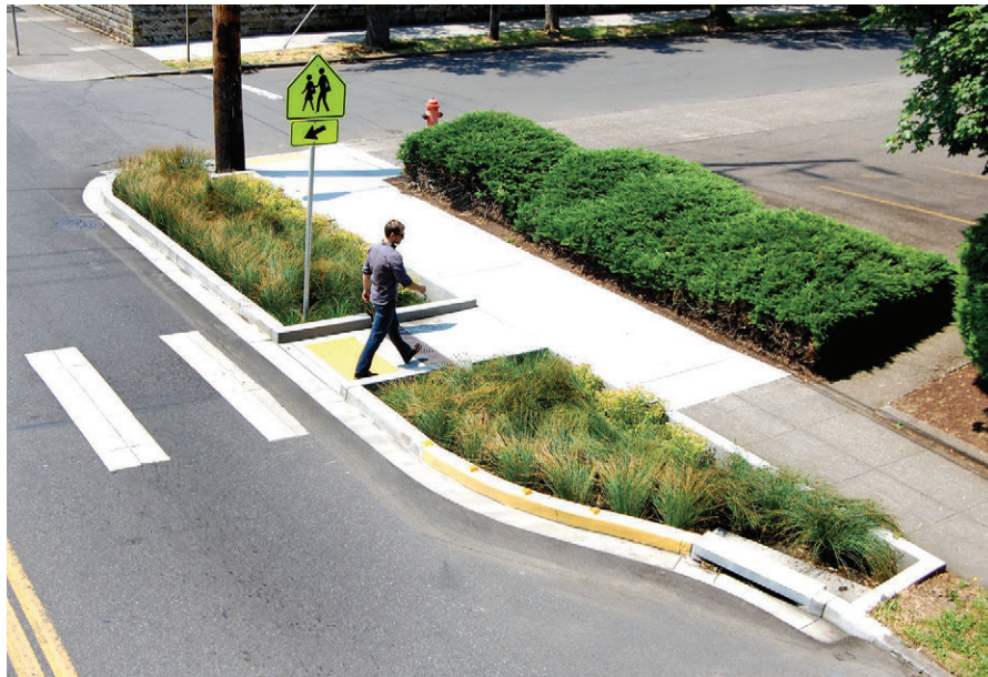
This GSI design treats runoff while guiding pedestrians safely to the crosswalk.
