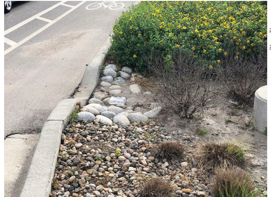
A sediment-clogged stone forebay.
