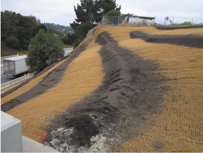
Compost filter berms placed perpendicular to slopes control stormwater velocity and provide filtration.
