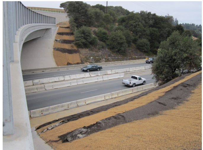
Compost filter berms placed perpendicular to the slope along the side of a highway.
