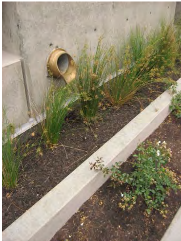
Figure 9. Disconnected downspout discharging to planter box.
