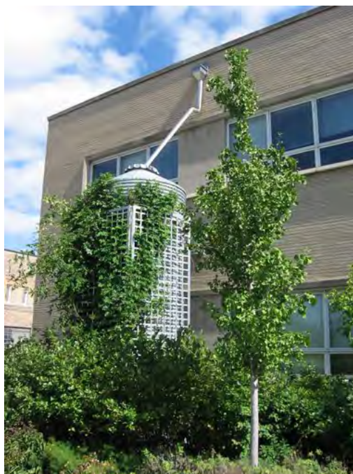
Figure 5. Rain water cistern.
