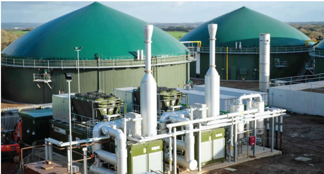
Figure 3.3. Picture of an Anaerobic Digester 21
