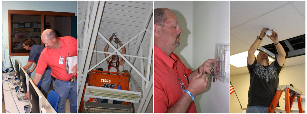
Improvements at Colorado's Coal Ridge High School. From left to right: Double-checking that computers are shut down, undergoing a lighting retrofit, turning off fans at the end of the day, and installing occupancy sensors in classrooms.
