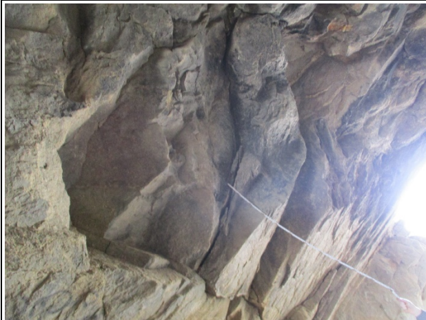
Condition State 4 Large unstable rock block
