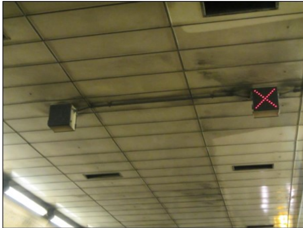
Condition State 4 Inoperable LUS
