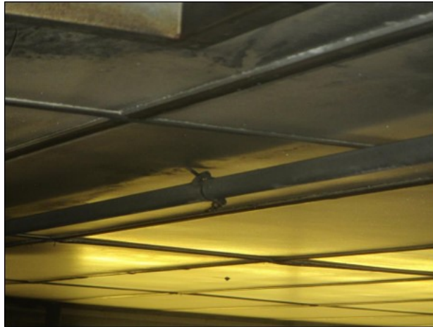
Condition State 2 Loose conduit anchorage
