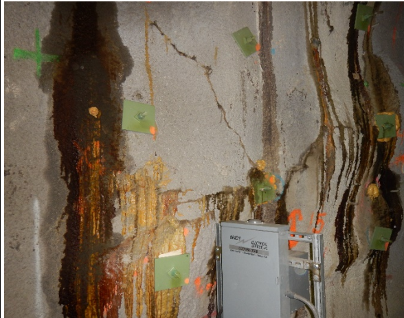
Condition State 3 Leakage with a saturated surface
