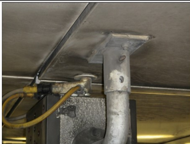
Condition State 3 Missing cotter pin at tubular ceiling bracket
