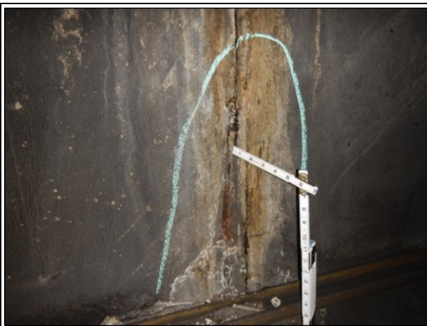
Condition State 3 Spall greater than 1" deep
