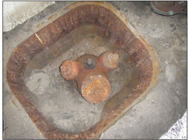
Condition State 3 Corrosion of hydrant
