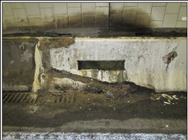
Condition State 4 Disintegrated barrier
