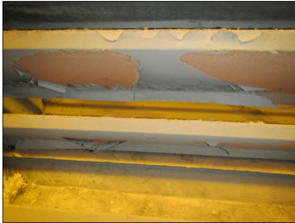
Condition State 2 Peeling coating and minor corrosion of louvers
