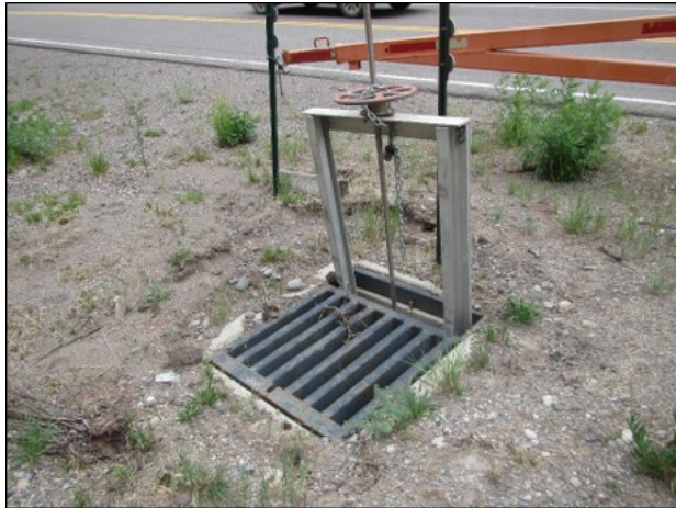
Condition State 2 Bent manual headgate
