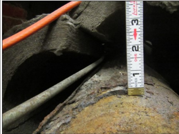
Condition State 2 Minor deterioration of water line
