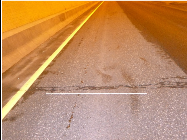
Condition State 2 Transverse cracking in the wearing surface
