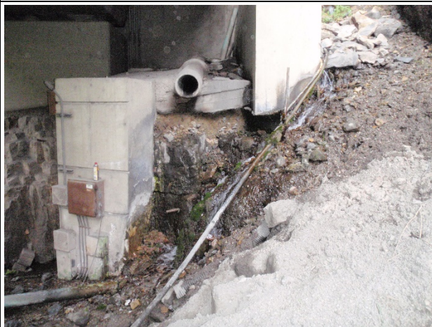
Condition State 4 Active leakage undermining portal
