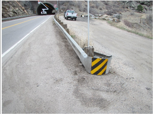
Condition State 3 Low end termination
