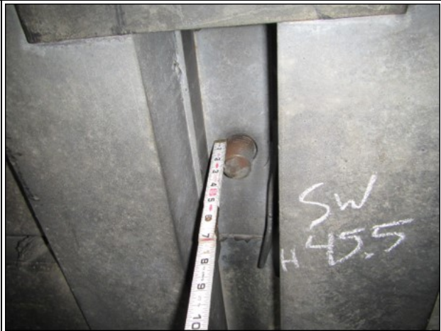
Condition State 3 Missing nut
