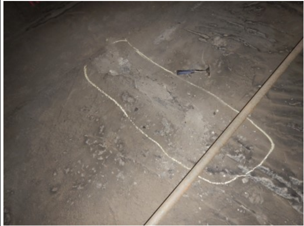
Condition State 4 Spalled membrane with exposed concrete
