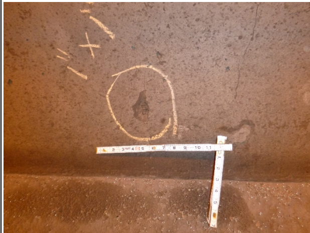
Condition State 2 Spall < 1" deep in the concrete barrier
