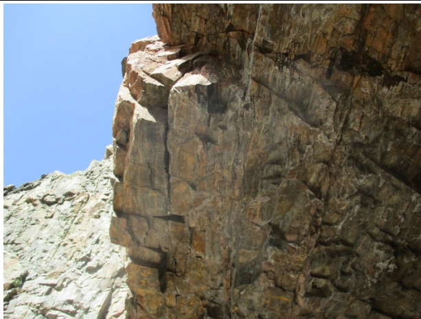
Condition State 3 Open joint at the portal
