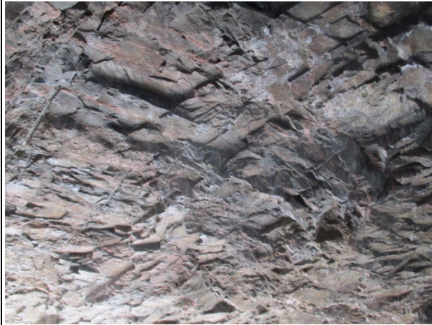
Condition State 2 Tightly interlocked rock blocks
