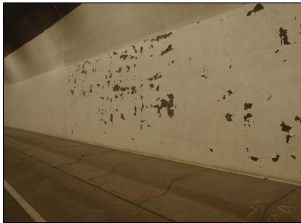
Condition State 4 Widespread failed coating
