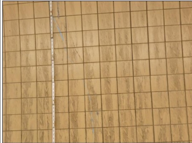
Condition State 2 Cracking without chipping or delamination
