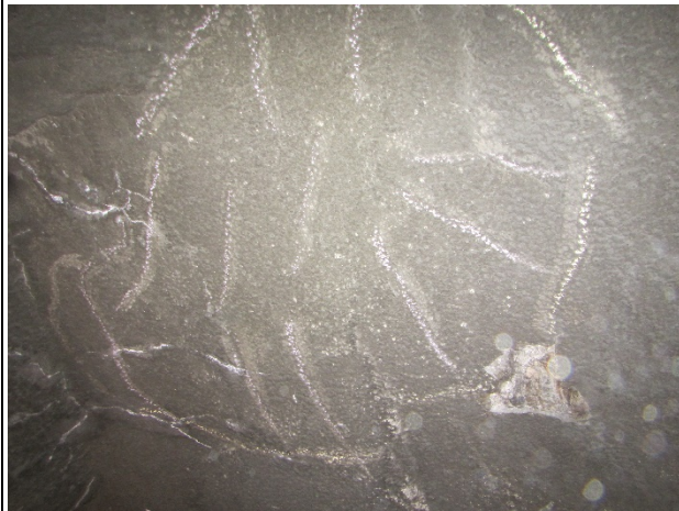
Condition State 2 Delaminated shotcrete
