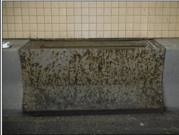
Condition State 3 Corrosion with minor section loss
