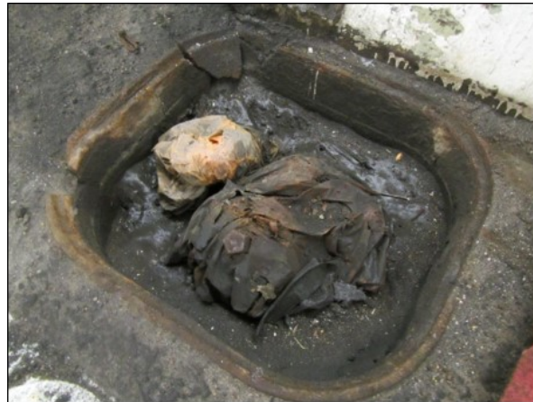
Condition State 4 Inoperable hydrant
