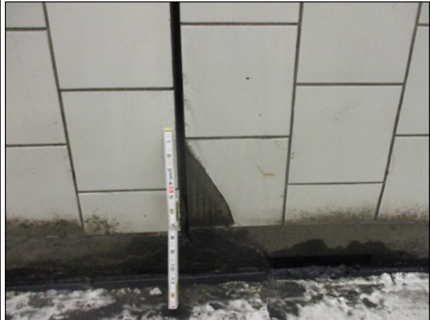
Condition State 3 Edge chipping of tile
