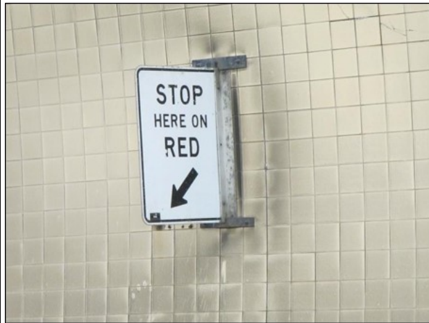
Condition State 1 Peeling lettering, legible (does not affect condition state)
