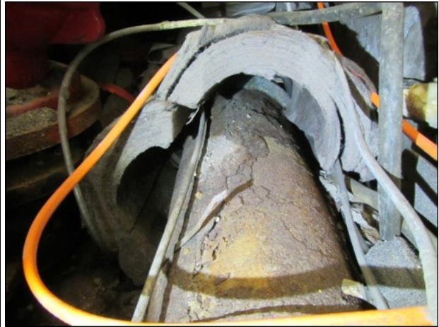
Condition State 2 Minor deterioration of water line with missing insulation
