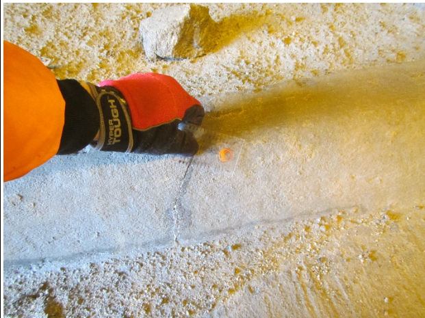
Condition State 2 Cracking in the concrete sidewalk
