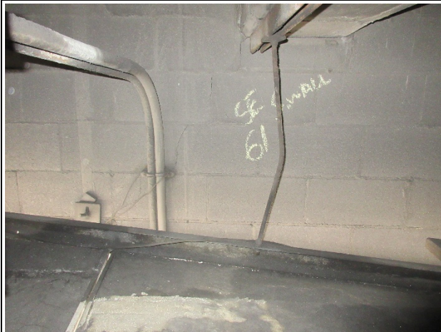
Condition State 2 Bowed hanger
