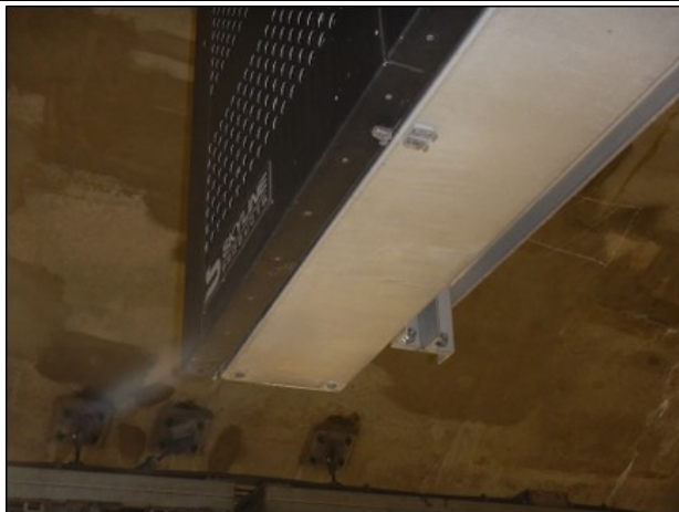
Condition State 3 Damaged housing and missing sign clips
