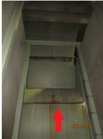
Condition State 2 Heavy corrosion of fan
