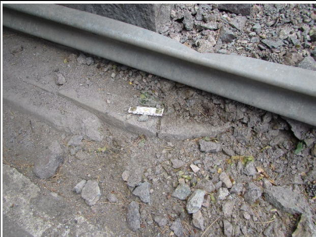
Condition State 3 Missing section at end of curb
