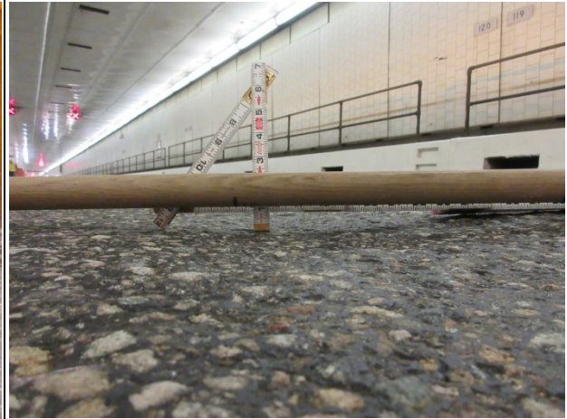
Condition State 3 Rutting in the wheel lines of the wearing surface
