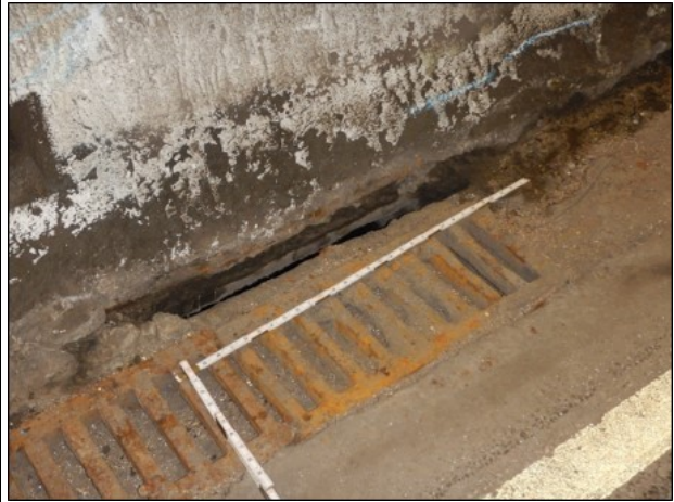
Condition State 4 Fully clogged roadway drain
