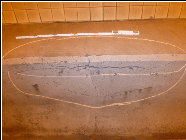
Condition State 3 Wide cracking near the top face of the barrier
