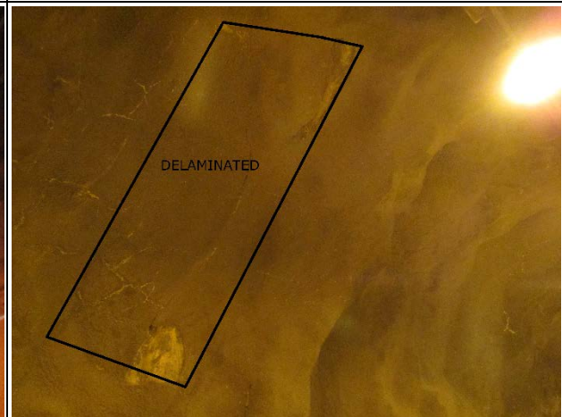
Condition State 4 Safety – delaminated and unstable shotcrete
