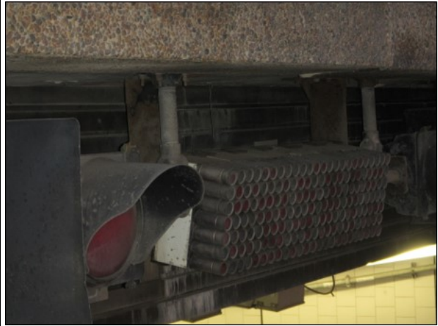
Condition State 4 Inoperable lane signal (stop light)
