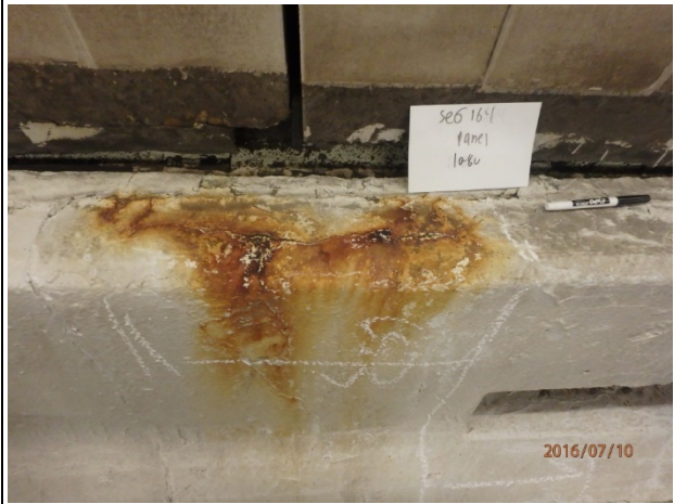
Condition State 3 Rust staining in the top face of the barrier
