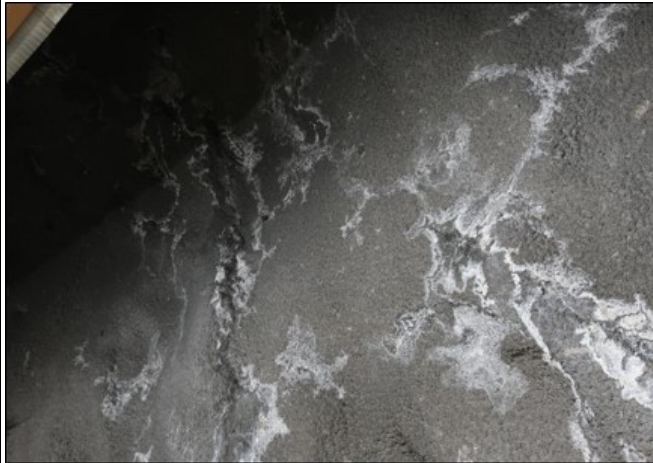
Condition State 2 Hairline cracking with efflorescence
