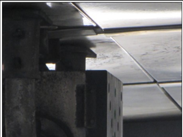
Condition State 3 Loose anchors and connection
