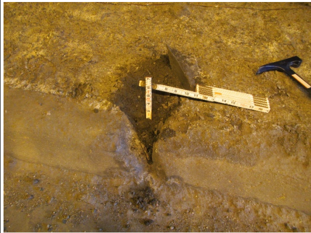
Condition State 3 Deep spall in the concrete curb
