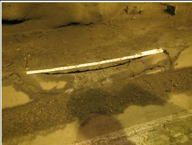
Condition State 3 Fully deteriorated concrete curb
