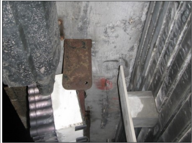
Condition State 3 Corroded connection brackets
