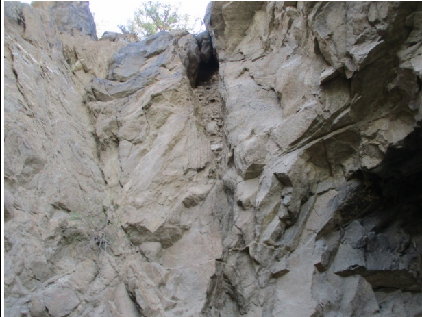
Condition State 3 Loose rock in the approach embankment
