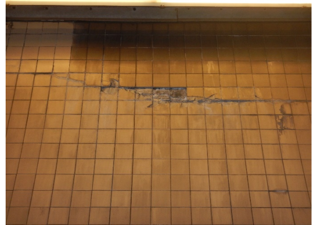
Condition State 4 Missing tile
