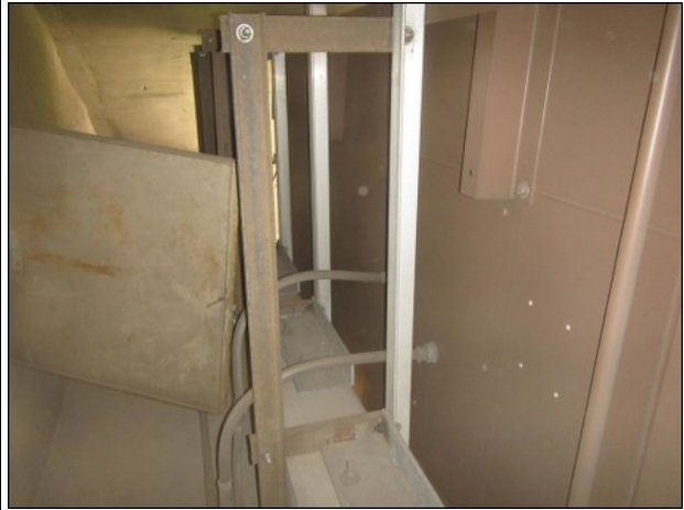
Condition State 2 Light corrosion of anchorage
