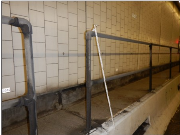
Condition State 2 Railing out-of-plumb (minor tilt)
