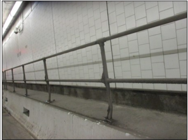
Condition State 3 Railing distortion requiring mitigation
