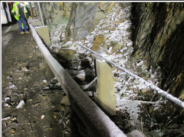
Condition State 4 Missing rail posts and damaged rail
