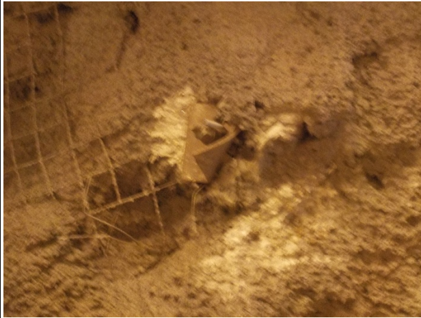
Condition State 2 Impact damage to bolt plate
