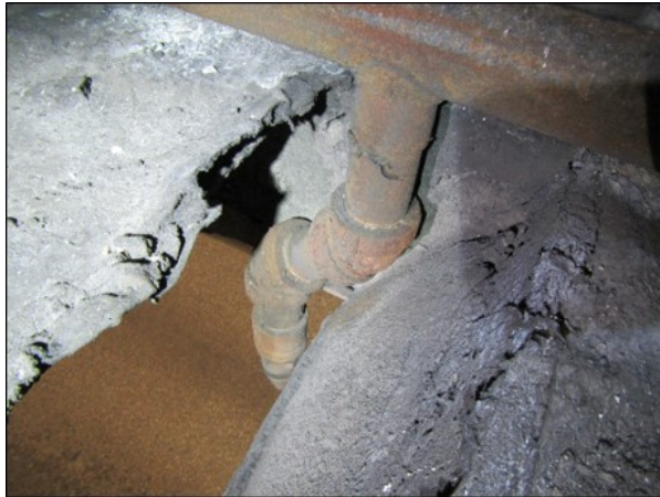
Condition State 2 Corrosion of sprinkler supply lines
