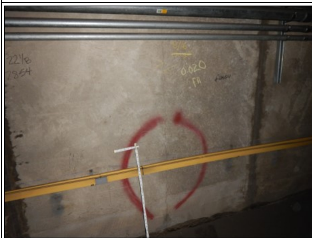
Condition State 3 0.02" wide cracking in prestressed concrete
