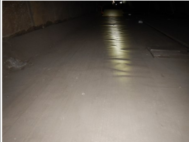
Condition State 2 Loss of adhesion of waterproof membrane
