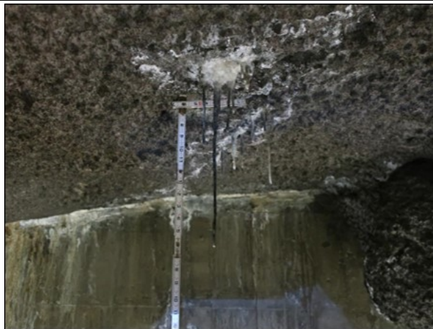
Condition State 4 Active dripping leakage
