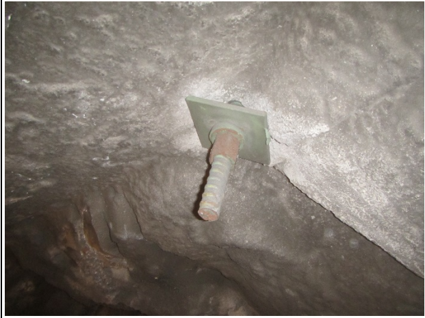
Condition State 2 Surface corrosion of rock bolt
