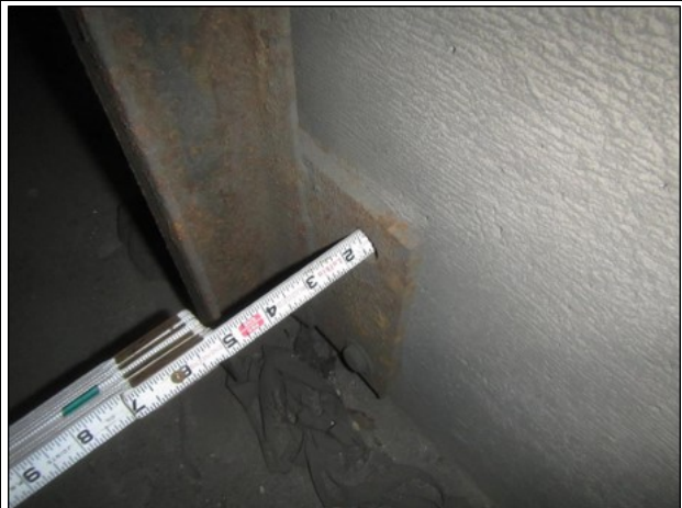
Condition State 3 Anchorage missing bolt
