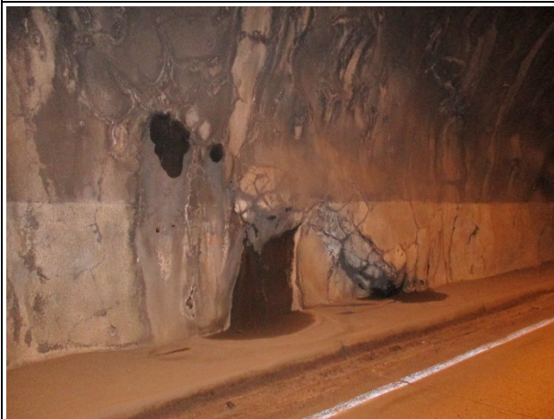
Condition State 4 Dripping leakage through the liner
