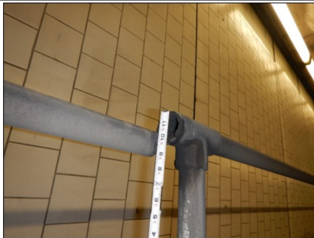
Condition State 3 Disconnected railing
