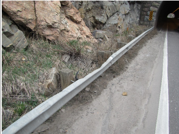
Condition State 3 Missing and split timber spacer blocks
