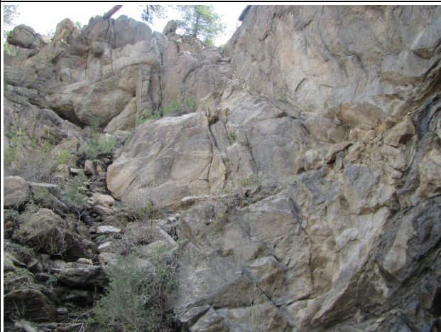
Condition State 4 Loose jointed rock with leakage
