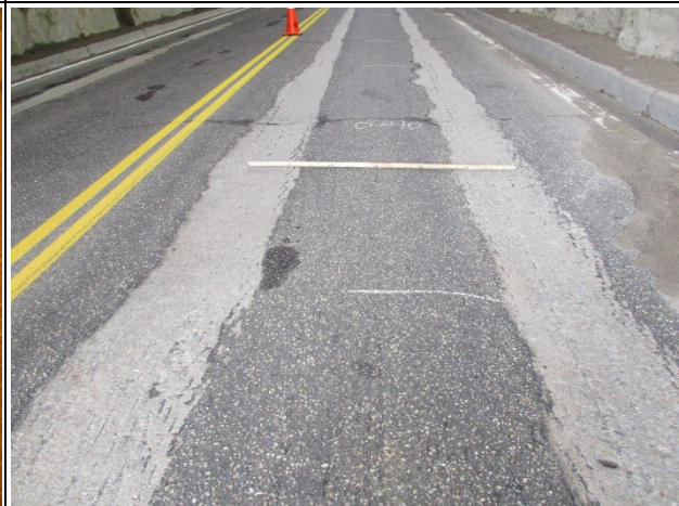
Condition State 4 Full depth rutting of asphalt wearing surface
