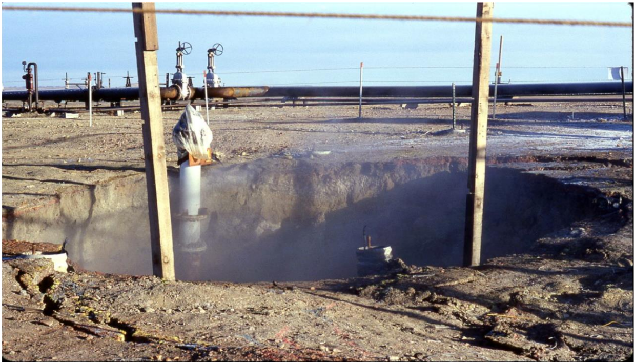
Figure7. At Hoe Creek, Wyoming, the cavity experienced a massive chimney collapse that propagated approximately 40 meters to the surface several weeks after the well was shut-in (LLNL, 2011).
