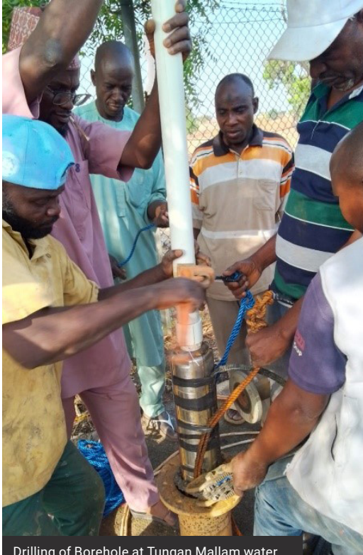
Drilling of Borehole at Tungan Mallam water station remote site © UN-Habitat/ Emmanuel Adeleke
