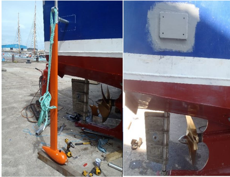
Figure 7 Attachment of the Hydropod to the vessel during drydock for underwater camera adjustment.
