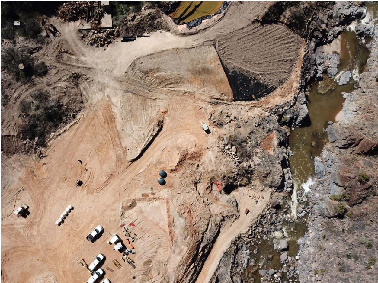
Figure 4-1. Aerial view of legacy mine remediation activities on Boulder Creek (15030202-005A) which was delisted for beryllium, copper and pH and manganese.
