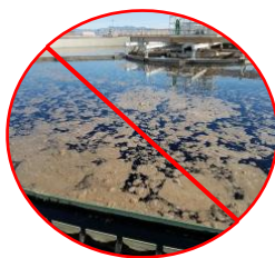
Scum floating in clarifier
