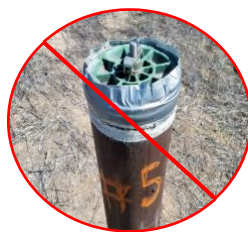
Poorly sealed POC well
