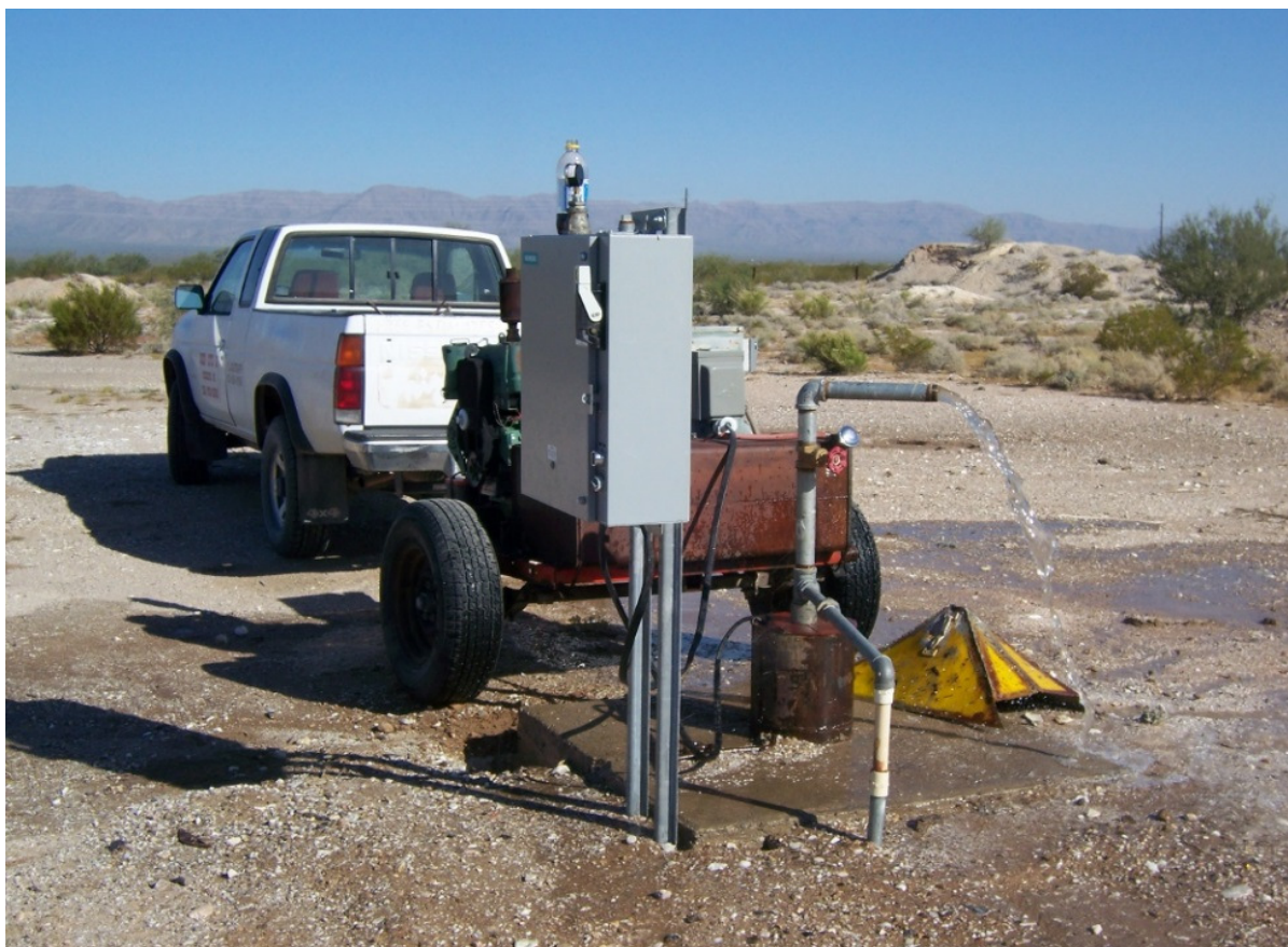
Figure 7 - Purging is especially important for intermittently used stock wells.
