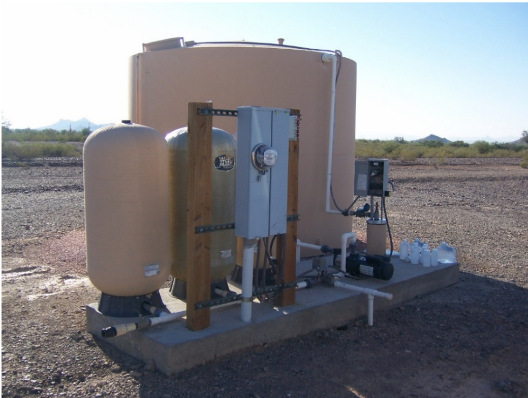
Figure 3 - Public water systems supplied by wells serve communities throughout the state.
