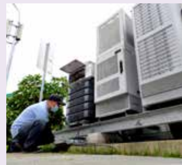
StarHub Mobile Base Station
