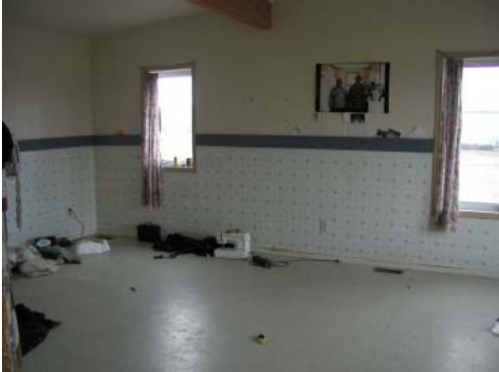
Figure 34. Linoleum flooring fastened to walls to protect them from damage by children.
