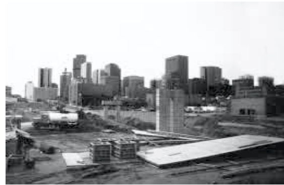
Courtesy of C. Galley
