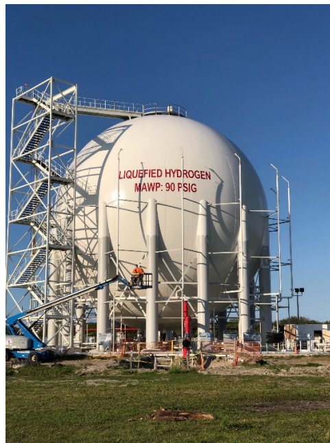
Figure 1. New NASA LH 2 Storage Tank After During Painting (Courtesy CB&I)
