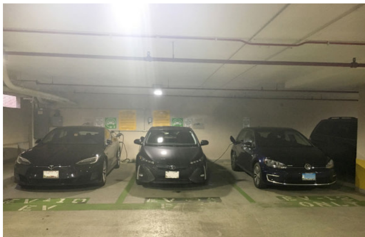
NIH'ers can charge their personal EVs at stations like this one in MLP-7, near the Lister Hill Center on the Bethesda campus.
