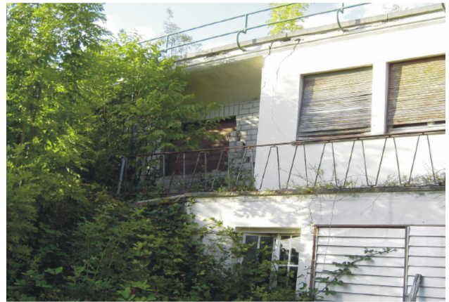
Fig. 2. Residential house in Reutlingen (Swabian Alb) damaged by a landslide (Blöchl and Braun, 2005).
