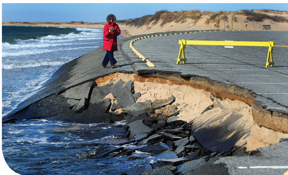
Damage to coastal roads is already a problem along the shores of the U.S. and will worsen as sea level continues to rise.
