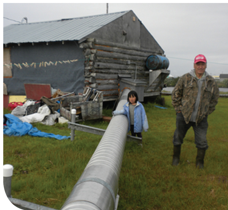
Rising temperatures are causing damage in Native villages in Alaska as sea ice declines and permafrost thaws. Resident of Selawik, Alaska, and his granddaughter survey a water line sinking into the thawing permafrost, August 2011.
