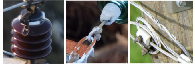
Figure 6: Small faults on power lines components (from left to right): cracked insulator, missing splint, broken wire.
