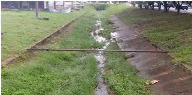
Figure 1 Poor drainage system.
