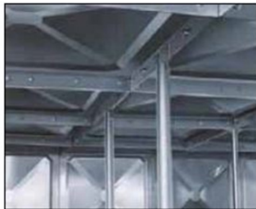
Figure 5 Protection from corrosion by choosing the right material.
