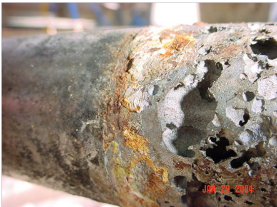
Figure 2 High Corrosion in water cylinders.
