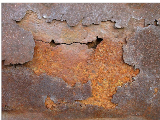
Figure 3 High Corrosion in Steel portable water cylinder.
