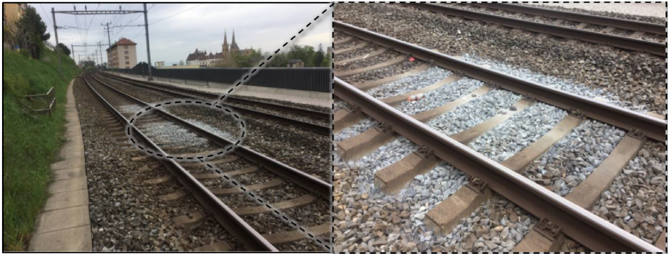
Fig. 1 White spots of ballast breakdown due to voided sleeper
