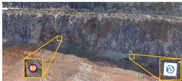
Figure 7: The reference point network allows an extensive accuracy evaluation. Systematic deformations of the image block and reconstructed object geometry can be quantified. Markers (bottom right) indicating GCP positions are shown in green, circular targets (left) for quantitative evaluation are in red.
