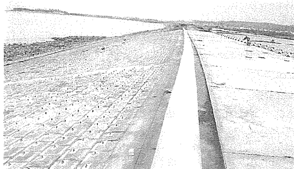
Figure 2. A section of seadyke in Hai Phong destroyed by the 2005 storms has just been consolidated with the cost of nearly 20 billion VND (1,250 million USD)
