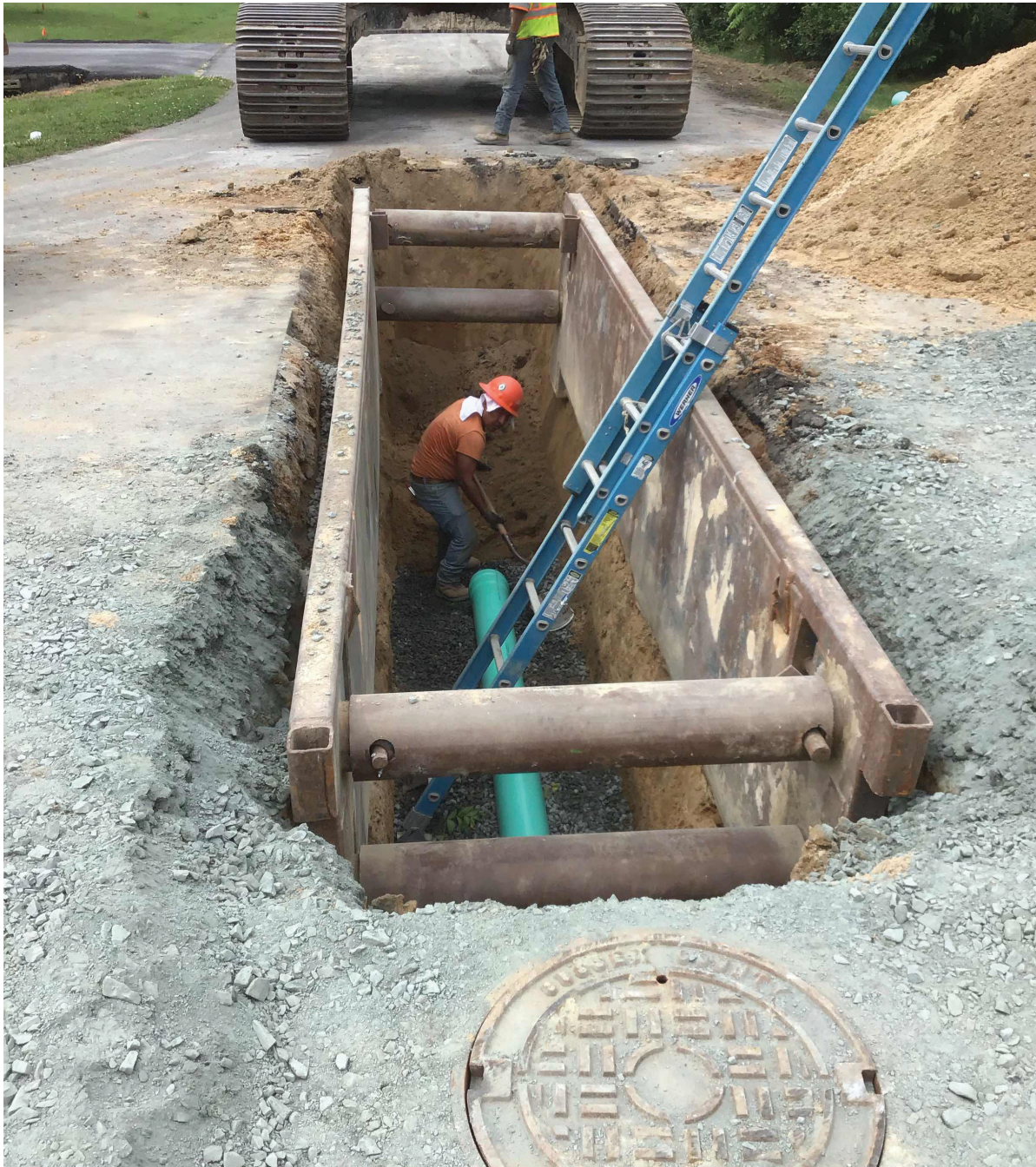
Sussex County contractors installing central sewer pipes. Photo courtesy Sussex County Government
