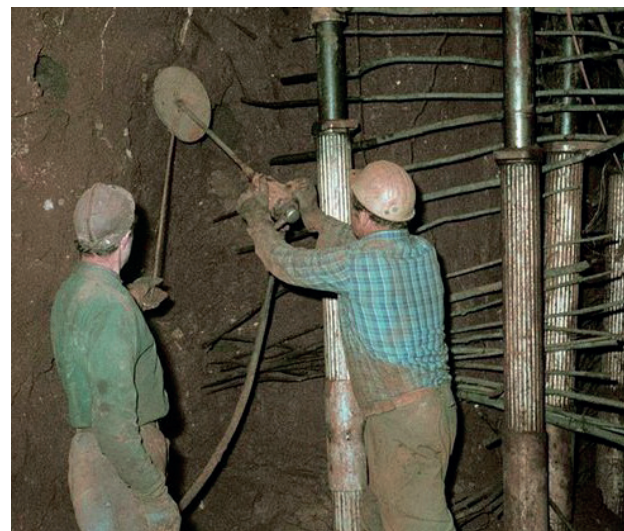
The drilling bit runs through a metal plate that is pressed against the wall by a 2nd miner for dust-prevention purposes.
