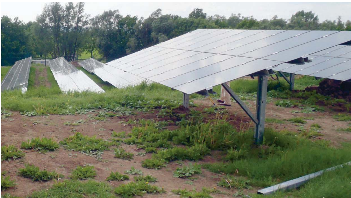
PV on a former waste dump, Azewijn, The Netherlands
