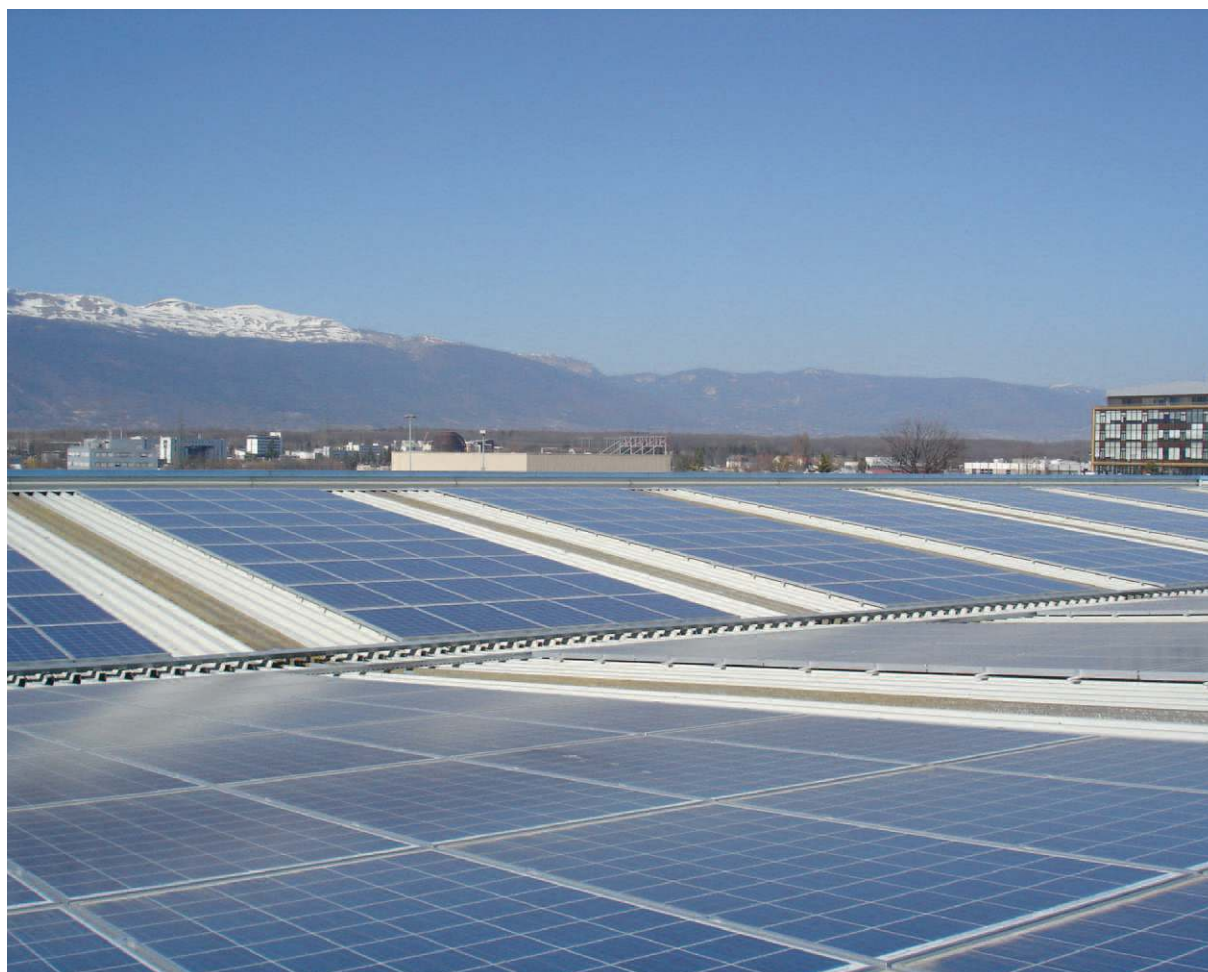
PV on a Brewery in Switzerland, Photo: ADEV Liestal
