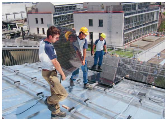
Roof-top installation in bern, Switzerland, Photo: BE Netz AG
