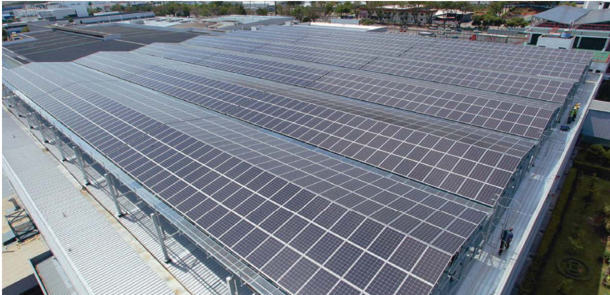
BIPV System at Bosch plant, Penang, Malaysia
