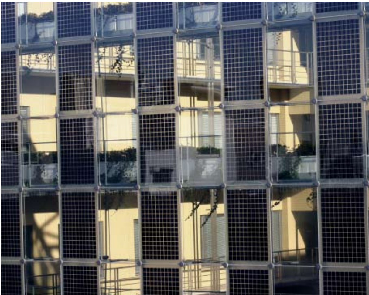
PV system at Kawasaki Municipal Tama Hospital, Japan
